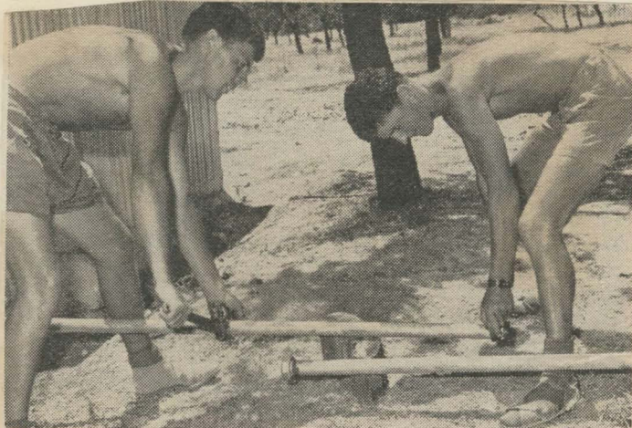
Installing a new water main at Limnitis. IRCON Engineers Sgt Michael Ahearne of Cork City (left) and Pte Gerry Walsh of Cappagh, Co Waterford will be glad to get the water flowing, 100°F makes piping hard to handle.
